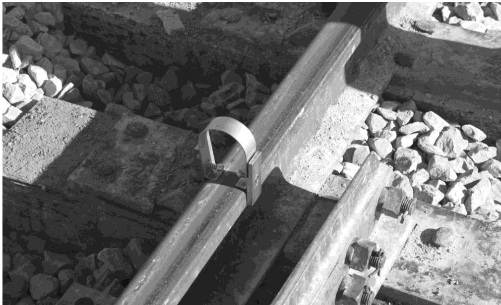
Figure 3.14 Gauge installed at the stock rail
